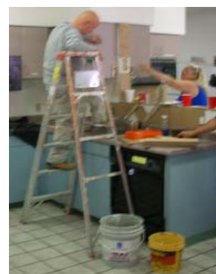
United Methodist Church Volunteers in Mission (VIM) from Bartlesville, OK work to re-tile our community kitchens.
