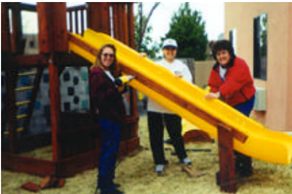
Bank of America volunteers Dana Kuck, Jamie Wilson and Francie Rawlins traded in their calculators and laptops for hammers and drills to assist with the construction of our new playground. The Bank also supported the project with a substantial cash donation.
